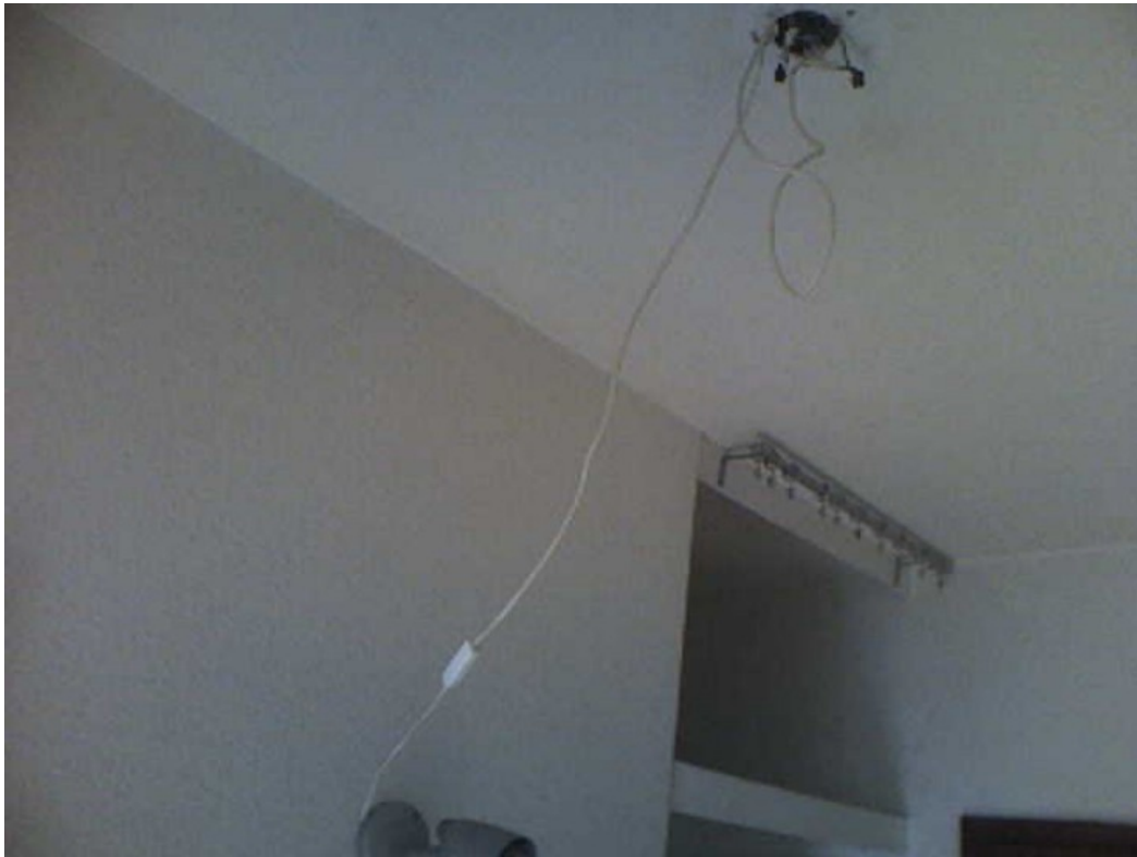
Exhibit B9 - Photograph depicting ceiling/fixture condition in accommodation.
